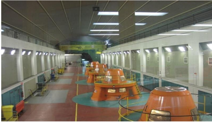
Tumut 1 Power Station
